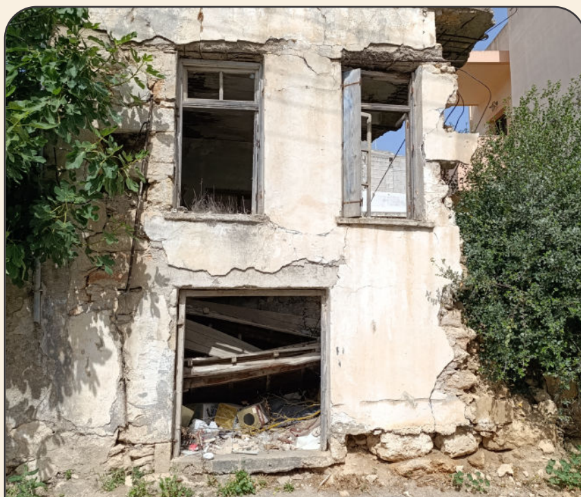
Facade of a house with cracked walls, damaged after an earthquake in Crete
